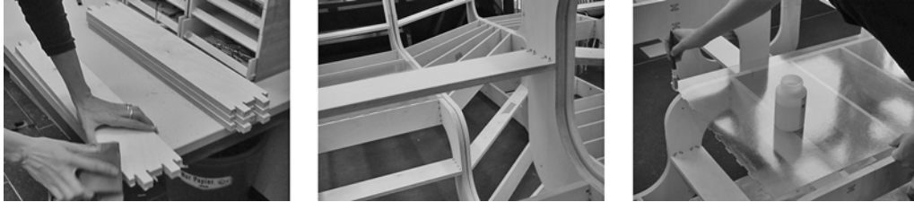
Figure 8. a) The edges of the milled plywood had to be chamfered manually; b) Mounted construction without the GRP; c) Toothed abutment of adhesive-fixed GRP sheeting
